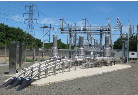
Commercial power distribution, Holbrook, NY
